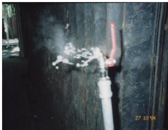
Figure 3.1 Steam at the pipe outlet
