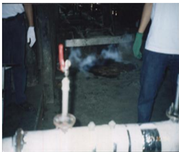
Figure 3.2 Visible high pressure steam from the inlet pipe
