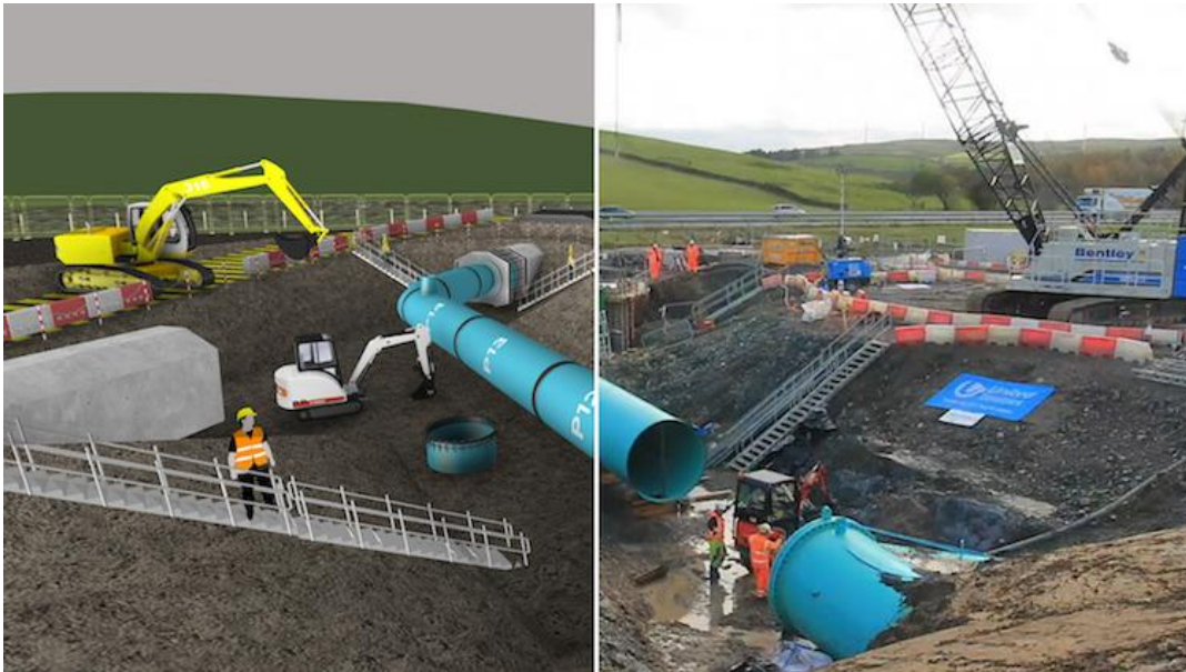
Figure 9: 4D in action: Mott MacDonald Bentley's pipeline project for United Utilities made huge time savings, image copyright of BimPlus
