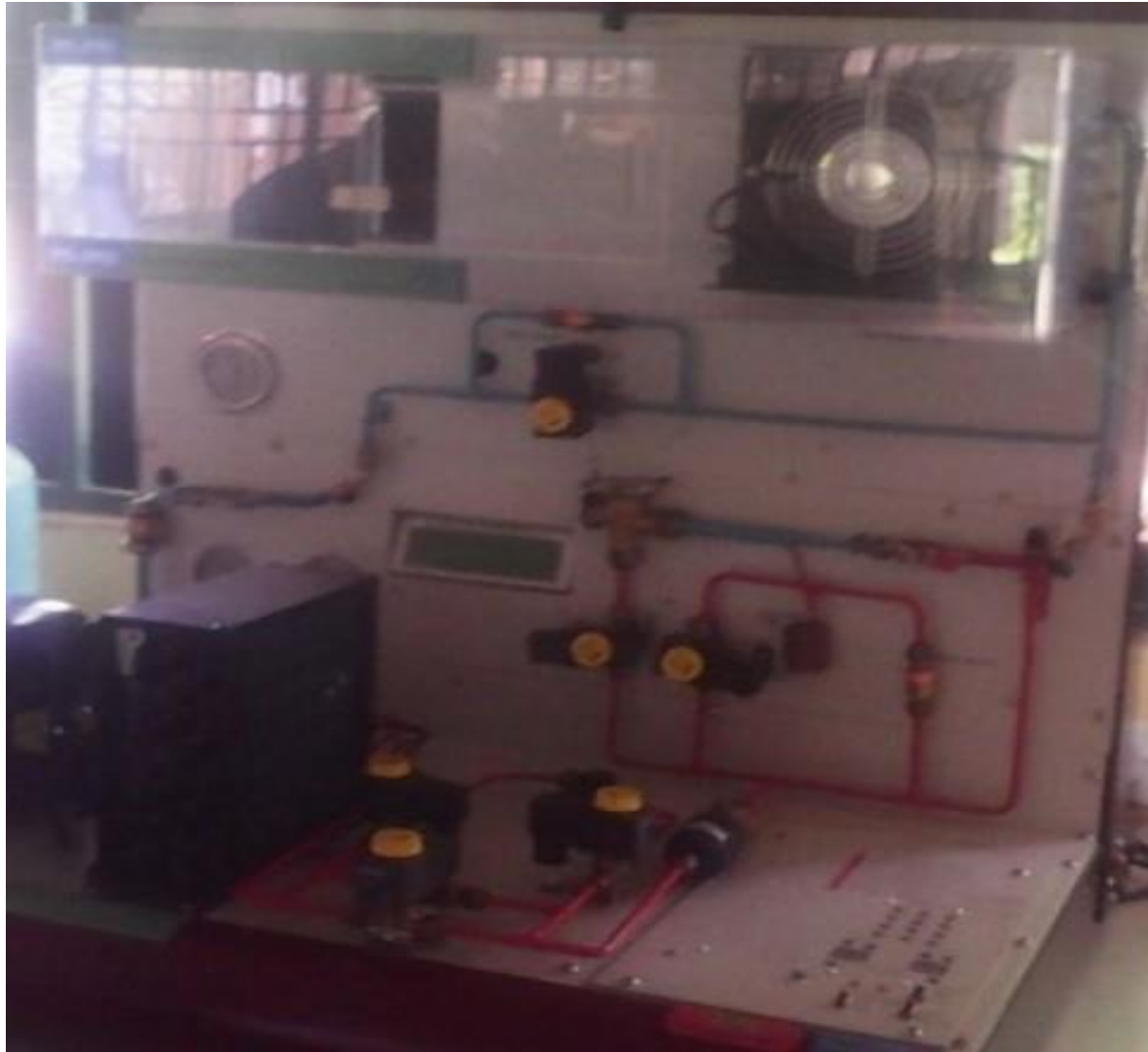
Plate 1.0: Theory Proving System for Air conditioning Unit
