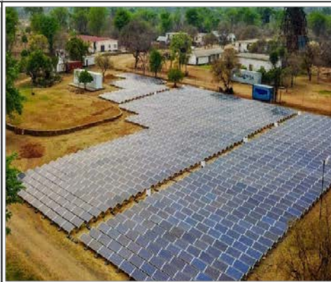
Figure 8b : 125K Wp installed by ENEO in Lomié (Eastern Cameroon)
