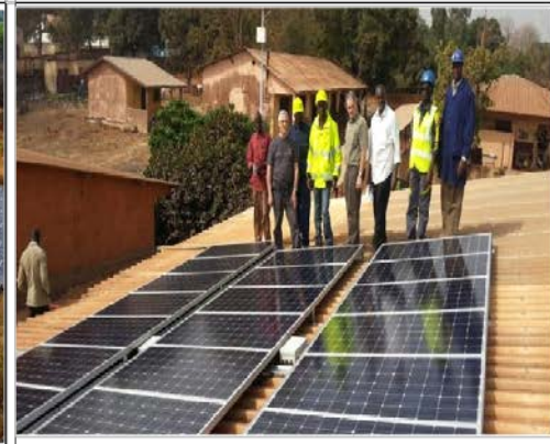
Figure 8c : Panel installed in northern Cameroon
