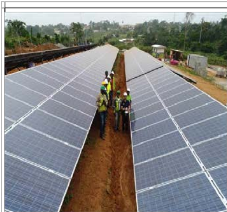
Figure 8a : 186K Wp installed by ENEO in Djoum (Southern Cameroon)
