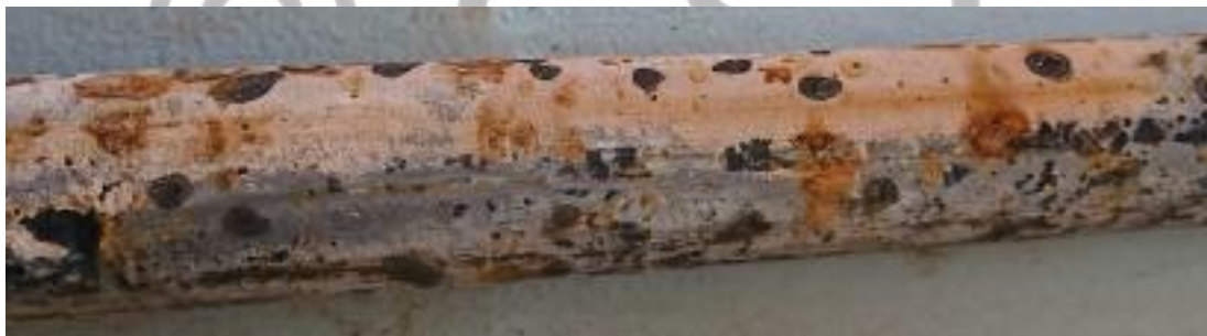
Fig.1: Rust for tube
