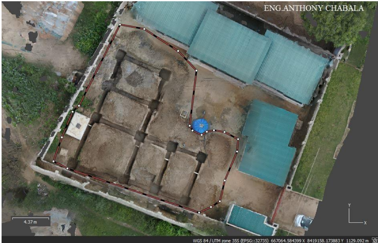
Figure 3: Orthomosaic image made from stitching of 296 JPG images captured from the drone for the foundation stage.
