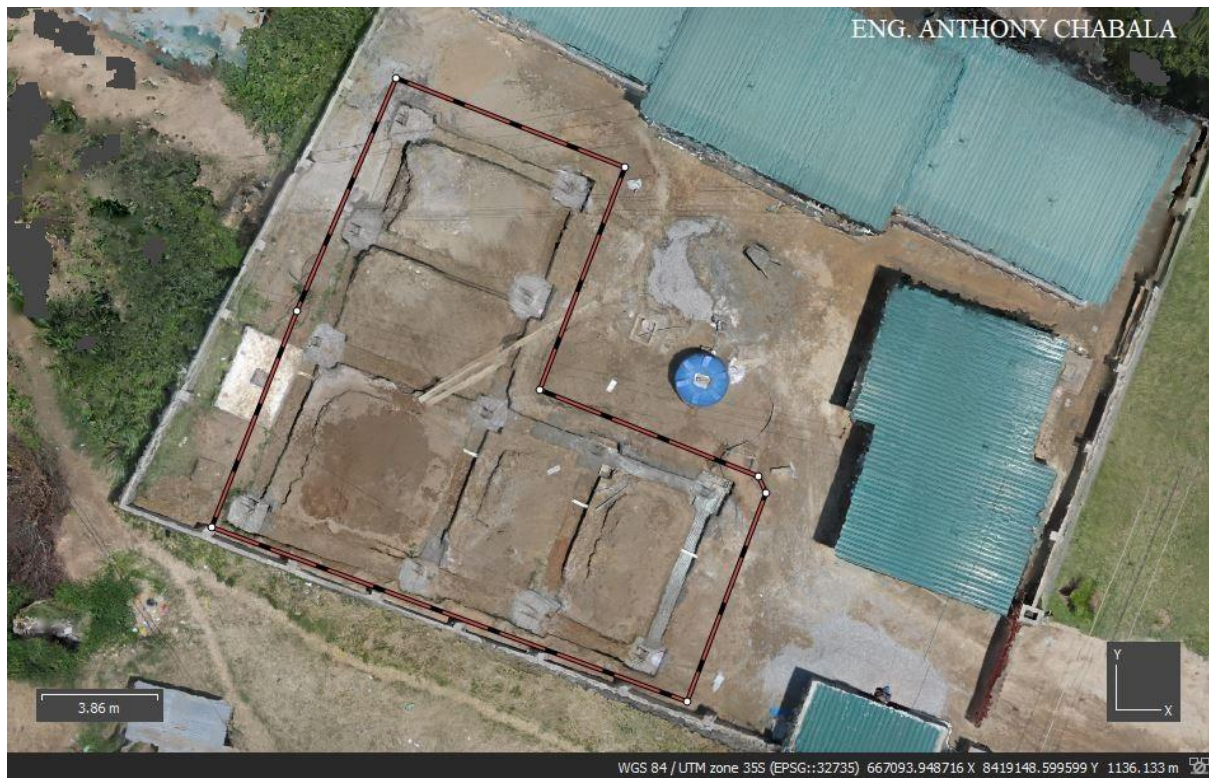
Figure 5: Orthomosaic image made from stitching of 166 JPG images captured from the drone for the footing stage.
