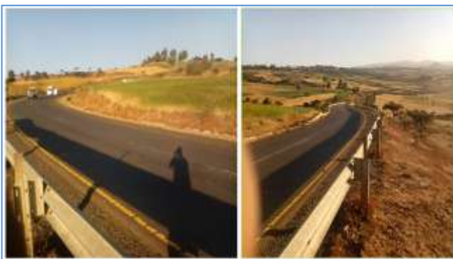
Figure 3.10 Miniinii Existing Road Condition
