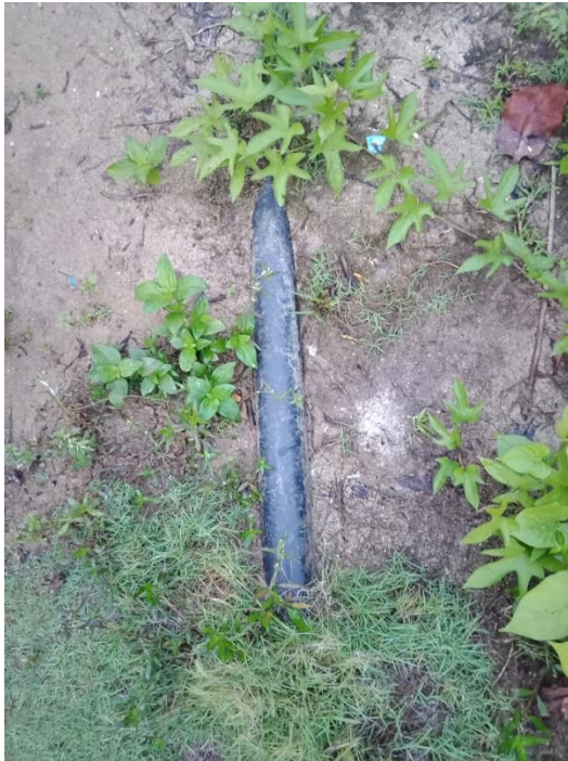
Photo 1: Ground Pipe (from upper of the river leading to the houses.
