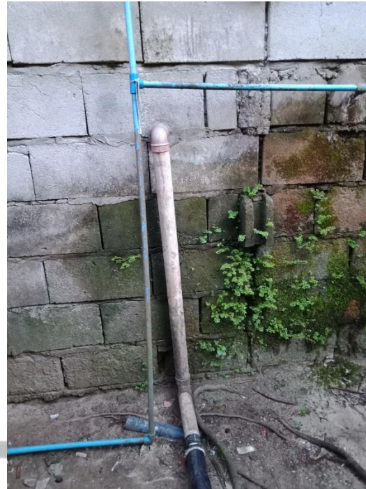
Photo 2: pipe entering the houses. Faucet are put to regulate flow.
