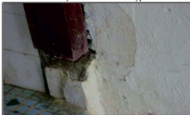
Figure 2: Concrete spalling at column area
