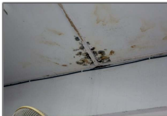
Figure 3: Areas of dampness in the ceiling
