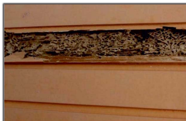
Figure 5: Broken doors and termite-infested doors.
