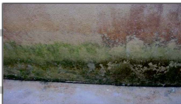
The Figure 1: shows mould and fungus growing on the wall of a toilet.
