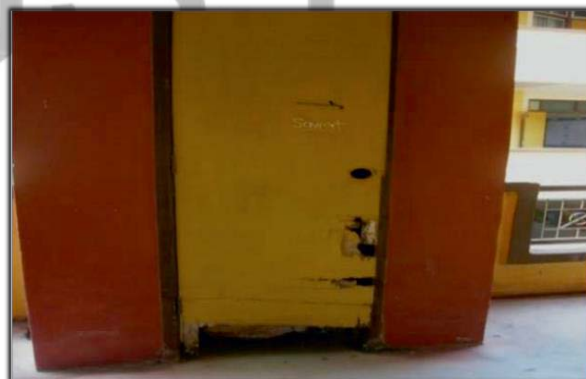
Figure 4: Some of the asbestos were broken
