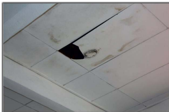
Figure 4: Some of the asbestos were broken
