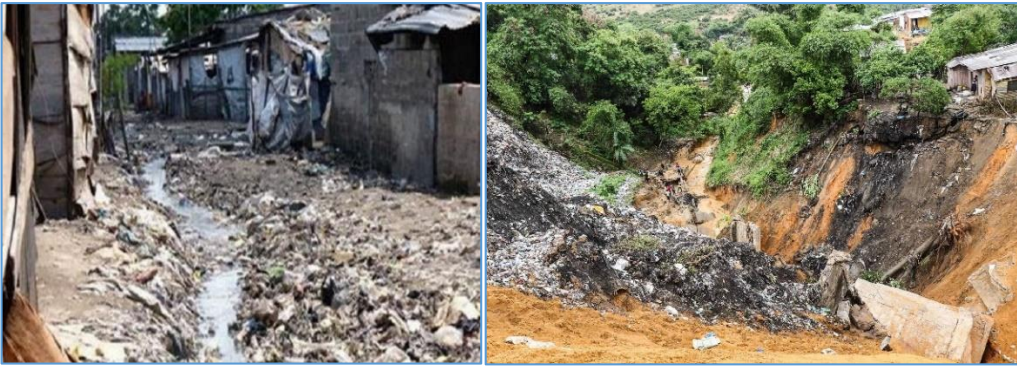
figure2(a and b): In the heart of downtown Kinshasa, causes of anarchic construction
