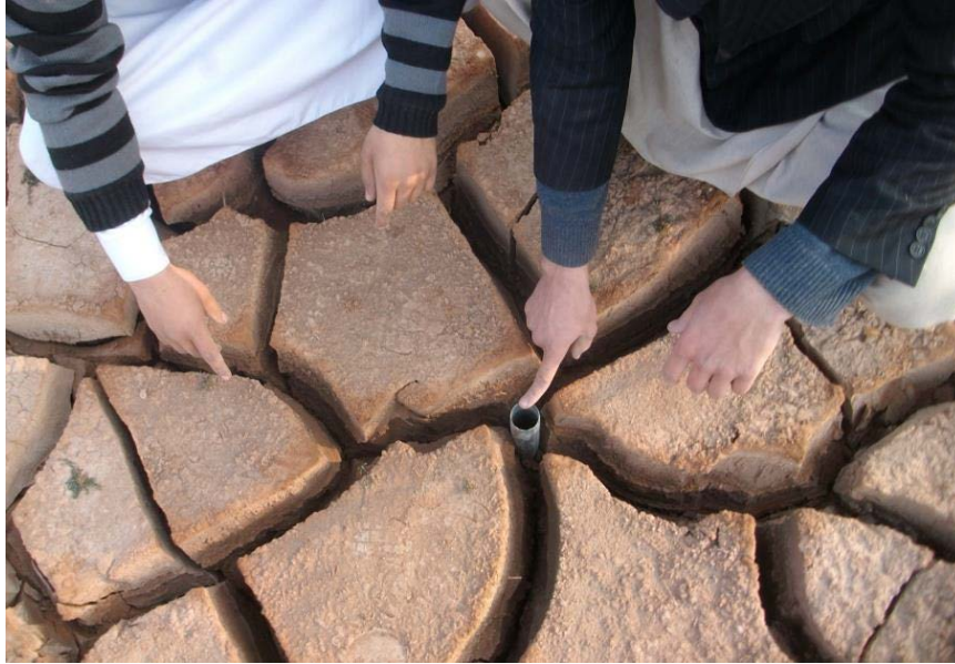
Figure 1. Expansive Soil Crack
