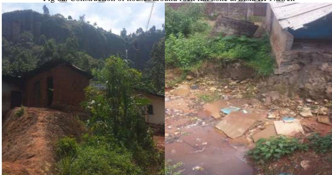
Fig 6b: Construction of houses on rocks and close to widening stream channel at Sisia
