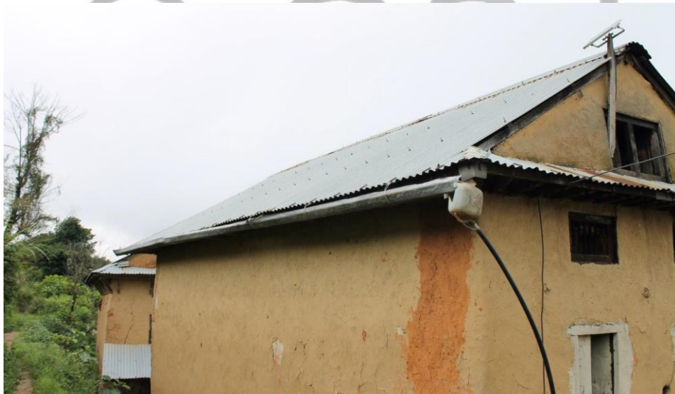
The proposed catchment area and gutter system for collection of rain water from traditional house`s roof
