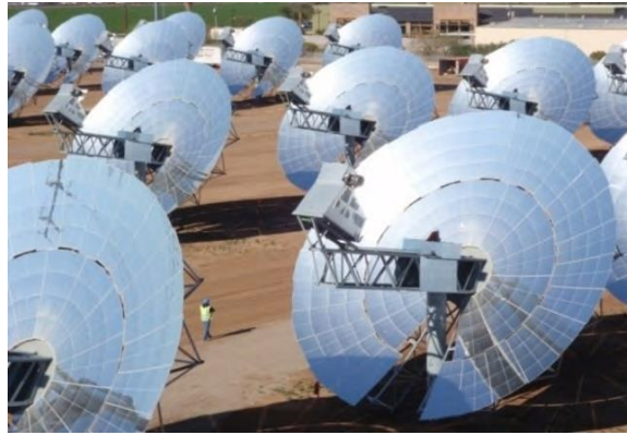
Figure 5-1: Solar panels in a power plant
