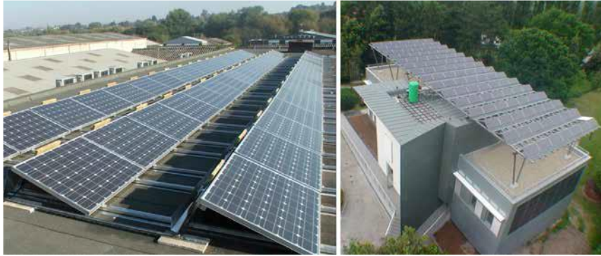
Figure8 Flat roof PV model and mini PV Farm
