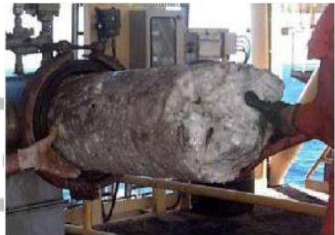
Figure 42: Hydrate formation in the natural gas pipeline [33]
